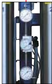
Differential Pressure Switch and Gauge
